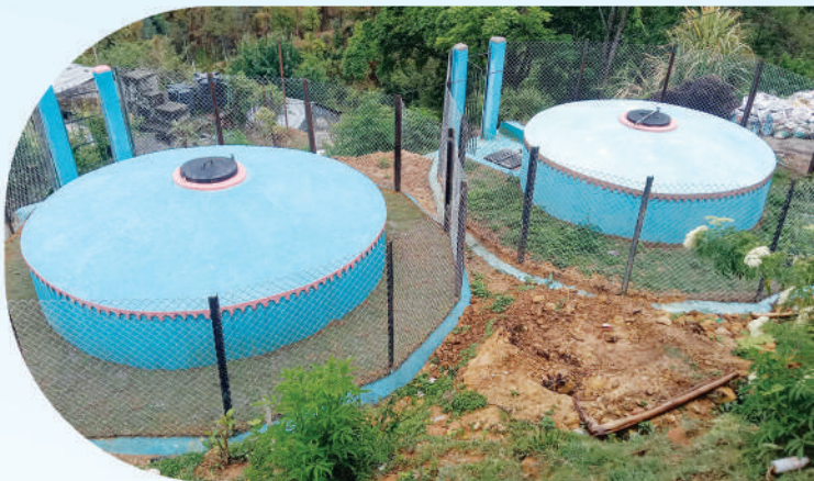
The Lapse Kotdanda Water Supply System served approximately 722 individuals living in 160 households
